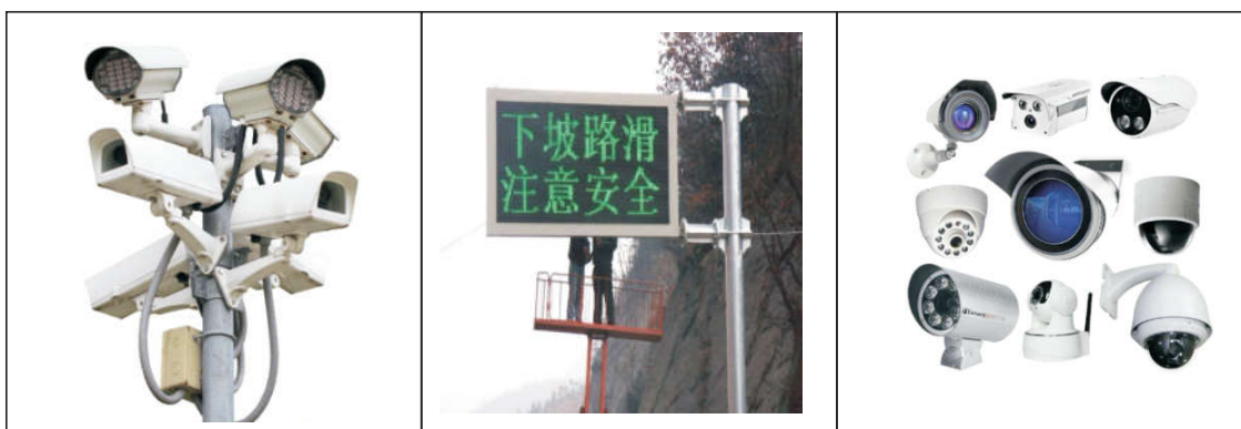
安防摄像设备 Security camera equipment
